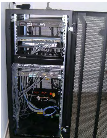
Vista general del Rack
