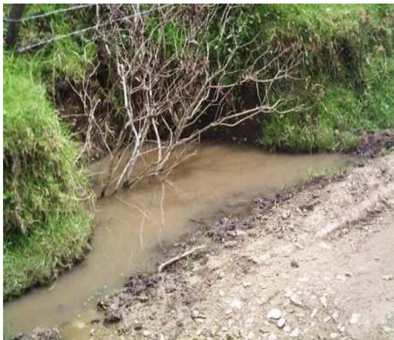
K 3+0500; N1 36.582 W77 00.412 Alcantarilla colmatada
