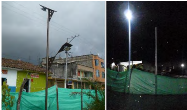
Figura 31. Luminaria led 50w poste 6m.
