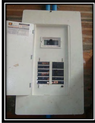
FIGURA 2.23. Colacteos Guachucal, tablero de breakers.
